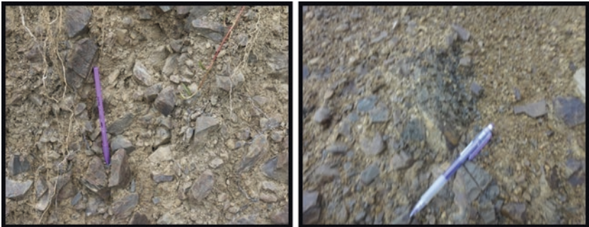
Fig. 12.6 Photographs showing the old landslide debris and colluvial deposit under Hakka-Myohaung Ward
