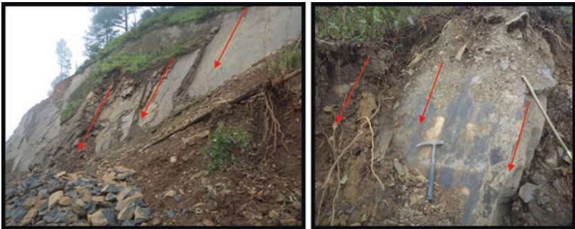
Fig. 12.9 Photograph showing slope failure along the Bedding Plane
